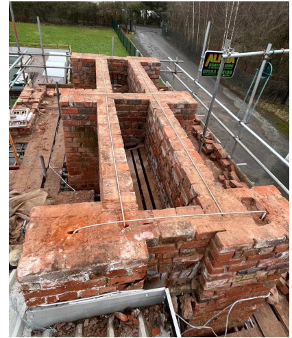
Top view of the northwest tower showing rebuilding before insertion of stainless steel ties and waterproof flaunching.
