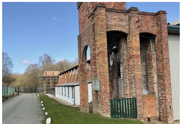
Full-length view of Hangar 16 showing the remedial work at the far end.
